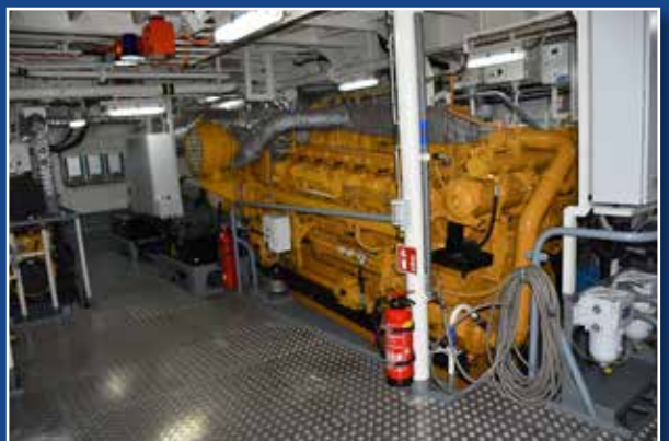
Starboard main engine
